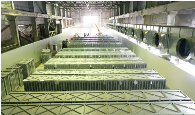
Moss Landing battery storage project is at the retired power plant site
