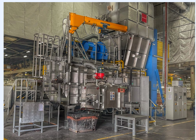
↑ New high efficiency aluminium melting furnace
